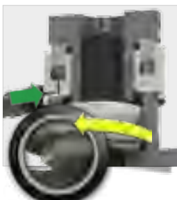
While the tool pressure is held, the hexagon nut is rotated down to the joint face and locked down tightly.
